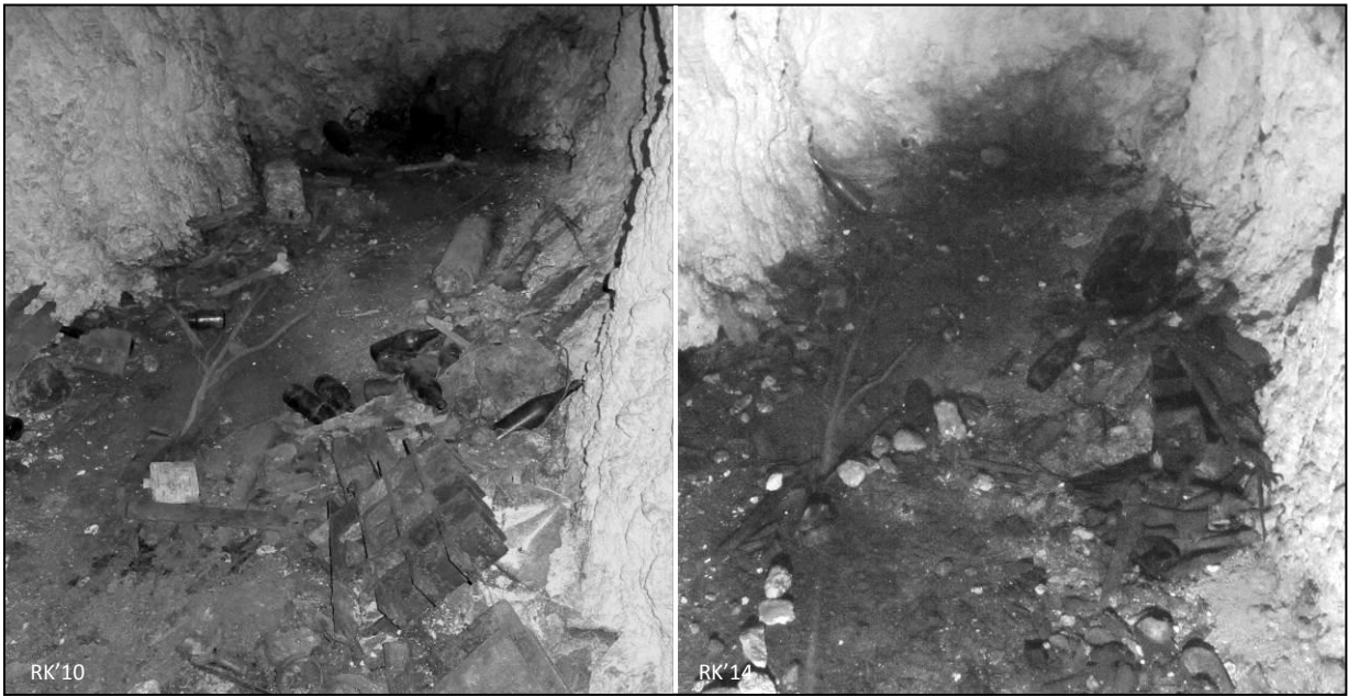
Figure 167 - AB98: cave interior showing disturbance to main assemblage and loss of wooden pigeonhole storage rack
