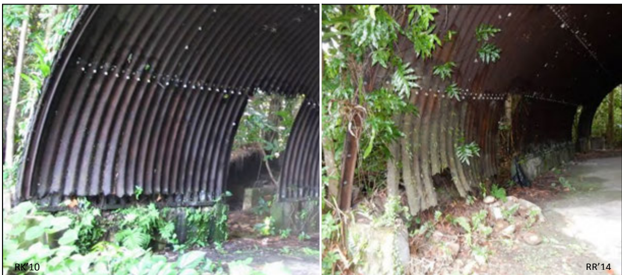
Figure 156 - AB38:2: American Motor Pool Quonset showing corrugated iron corrosion since 2010
