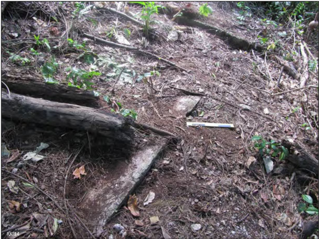
Figure 139 - AB14-072: concrete foundations bases eroding out of hillside
